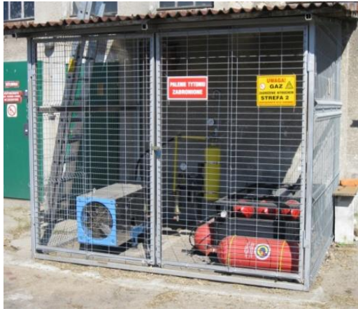
Gas compressing station
