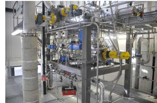
Continuous Steam Explosion reactor
